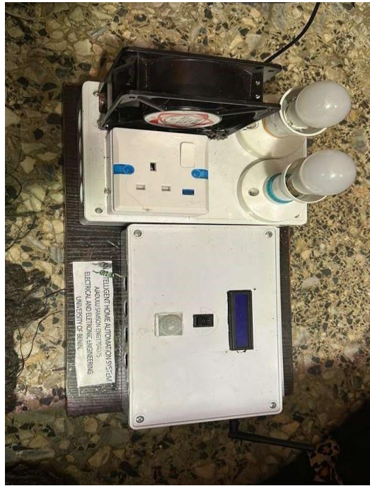
Fig. 8. Automated smart system (When Device is off)
